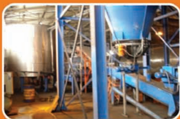
Factory inside view
