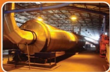
Factory inside view
